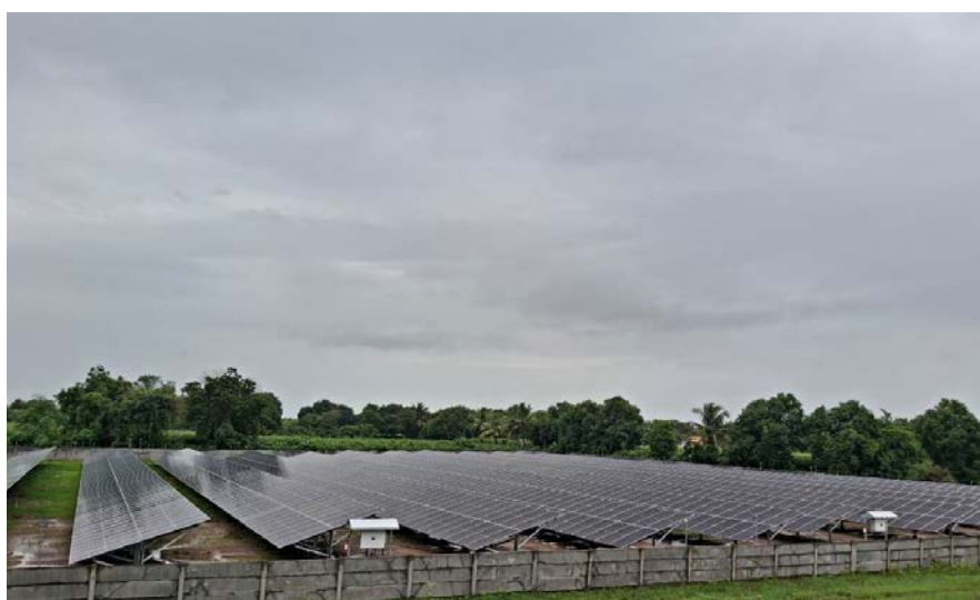
Solar energy infrastructure at the Group's manufacturing premises, reflecting its focus on building a more conscious and sustainability-led diamond ecosystem.
